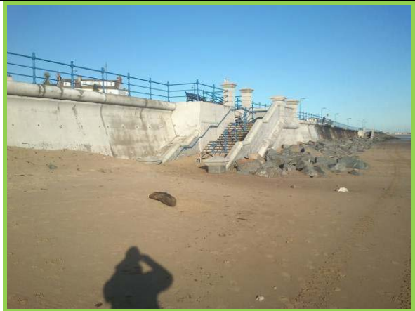
High sand levels at new southern set of steps, showing rebuilt section of wall next to new step structure. (Asset Ref. No. 1221C901C0501C05)
