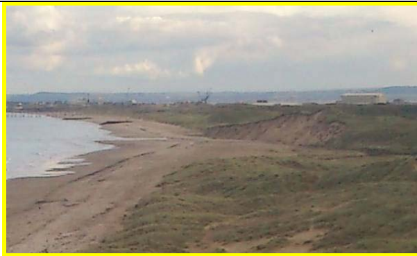
Crimdon beck in mid photo, showing steep eroding dune face where beck is close to toe. (Asset ref. No. 1221C901C0301C01)
