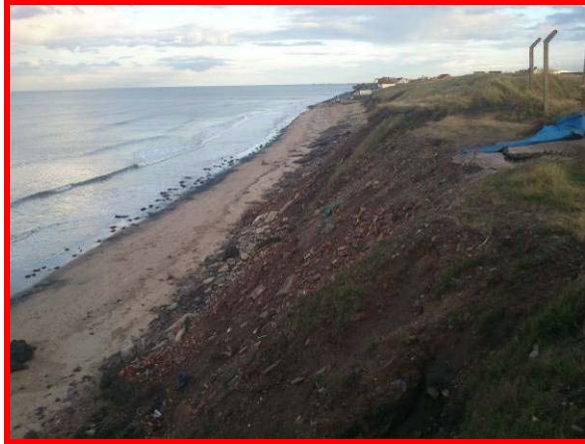
Eroding embankment cliff, previously protected by brick filled gabions which have failed. (Asset ref. No. 1221C901C0302C02)
