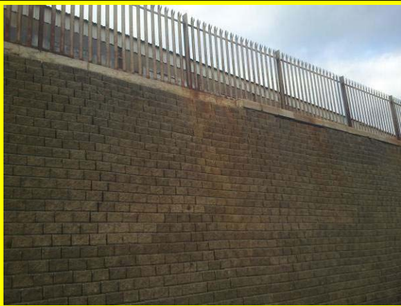
Missing coping stones and bulging of the wall. (Asset ref. No. 1221C901C0401C19)
