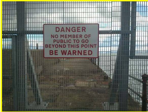
Fencing and warning signs at mid length of breakwater. (Asset ref. No. 1221C901C0401C01)
