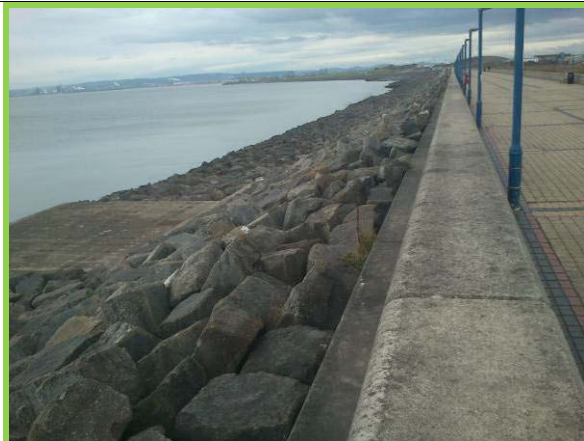
Rock armour defence in good condition to south of South Pier (Asset ref. No. 1221C901C0401C33)
