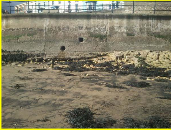
Low beach levels undermining wall near south of Block Sands reclamation. (Asset ref. No. 1221C901C0401C04)
