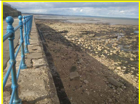
Damage to concrete coping units increases towards south. (Asset ref. No. 1221C901C0303C02)
