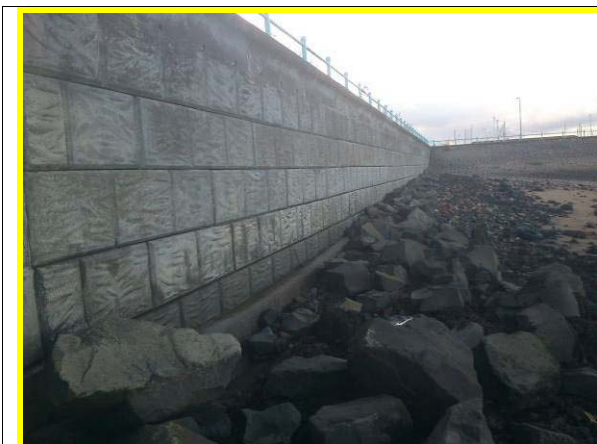
Rock armour at toe of wall looking west from steps (Asset ref. No. 1221C901C0401C27)
