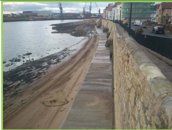
View of Town Wall from east end, showing new toe protection apron (Asset ref. No. 1221C901C0401C35)
