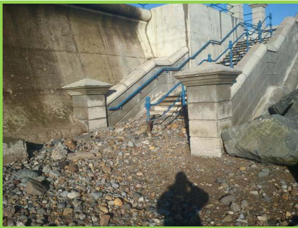
High cobble beach level adjacent to rebuilt northern steps. (Asset Ref. No. 1221C901C0501C05)
