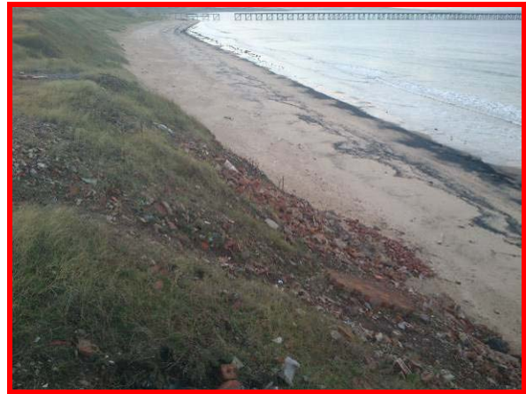
Eroding embankment / cliff previously protected by brick filled gabions. (Asset ref. No. 1221C901C0302C02)
