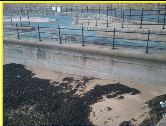
Block Sands seawall at north near Heugh Breakwater (Asset ref. No. 1221C901C0401C04)
