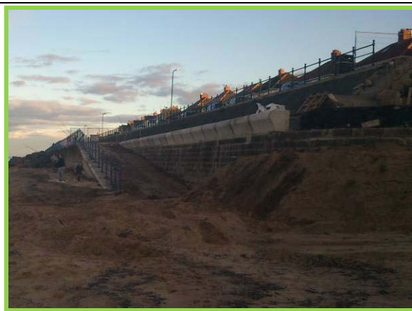
Works underway to replace sections of seawall at return end (Asset ref. No. 1221C901C0303C01)
