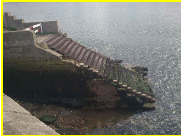
Steps at former passenger ferry landing at west end of town Wall, (Asset ref. No. 1221C901C0401C35)
