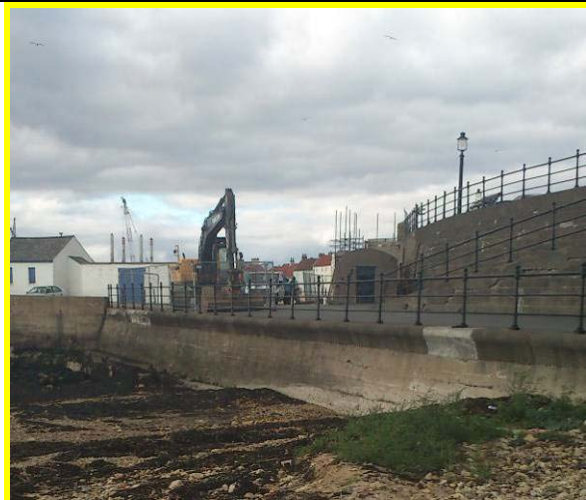
Repaired section of coping in foreground, further damage in distance (Asset ref. No. 1221C901C0401C05)
