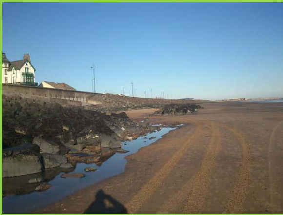
Rock armour beach control structures near Little Scar (Asset Ref. No. 1221C901C0501C05 foreground, 1221C901C0401C33 in distance)
