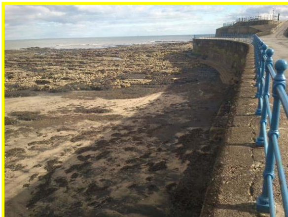
View of wall in fair overall condition, looking south (Asset ref. No. 1221C901C0303C02)
