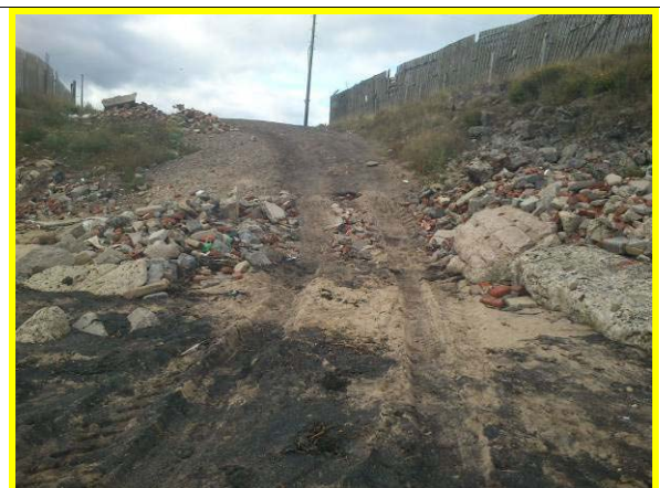
Informal beach access ramp with tipped demolition waste. (Asset ref. No. 1221C901C0401C18)
