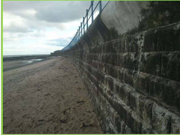
View of blockwork wall with repairs to cope. (Asset ref. No. 1221C901C0303C01)
