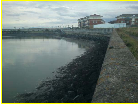
Rear flood wall at south part of West Harbour in fair condition. (Asset ref. No. 1221C901C0401C29)
