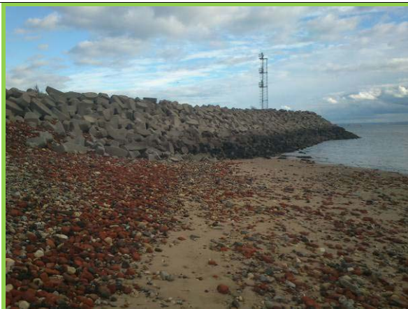
Middleton Jetty in good condition. Retains sand and rubble beach to south (Asset ref. No. 1221C901C0401C16)
