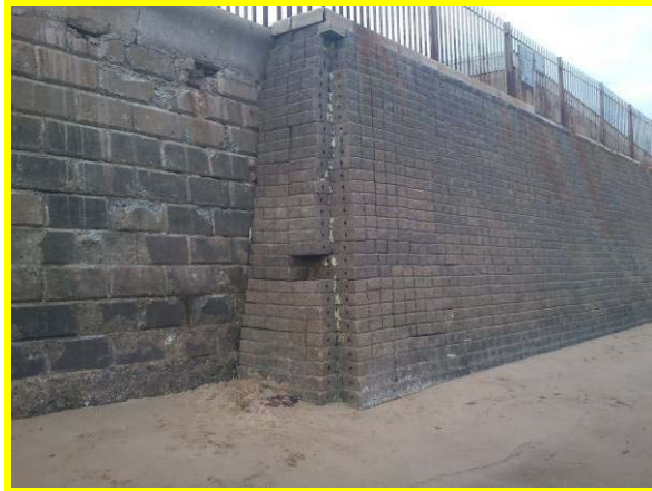
Missing blocks at interface between two sections of wall (Asset ref. No. 1221C901C0401C19)
