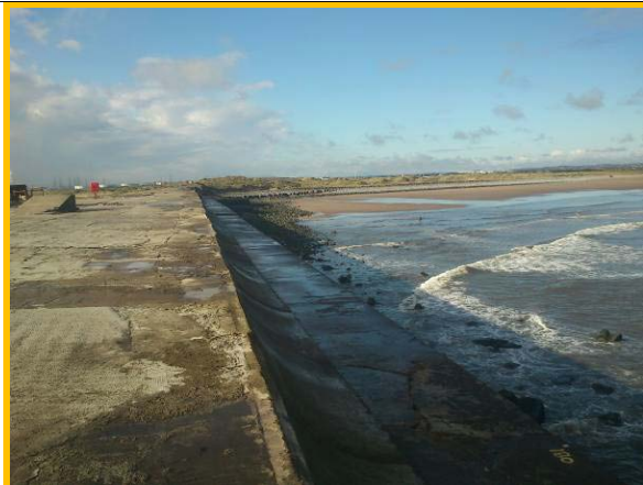
View of upper deck level showing patch repairs and northern side of breakwater from near fence. (Asset ref. No. 1221C901C0502C01)
