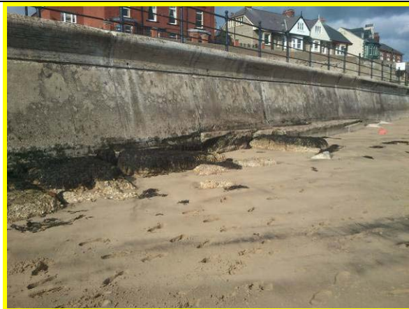
Toe scour and undermining towards south of Block Sands wall. (Asset ref. No. 1221C901C0401C04)
