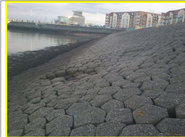
Area of settlement in block revetment (Asset ref. No. 1221C901C0401C25)
