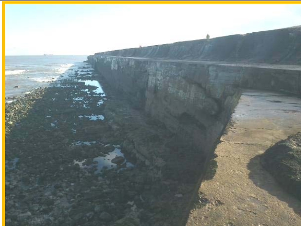
Northern side of breakwater, with extensive cracking and voids. (Asset ref. No. 1221C901C0502C01)
