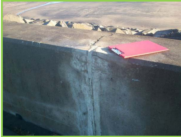
Construction joint in crest wall with failed previous repairs south of Newburn Bridge (Asset ref. No. 1221C901C0401C33)
