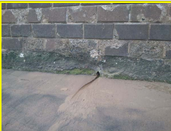
Older concrete block wall in foreground; newer slightly sloping smaller block wall in distance. (Asset ref. No. 1221C901C0401C19)
