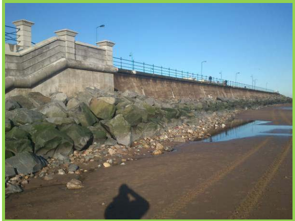
Northern set of steps has been substantially repaired / rebuilt since 2010 (Asset Ref. No. 1221C901C0501C05)
