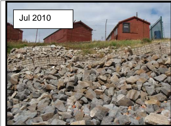
View of Gabion baskets with rock armour. Photo from 2010 report. (Asset ref. No. 1221C901C0401C17)
