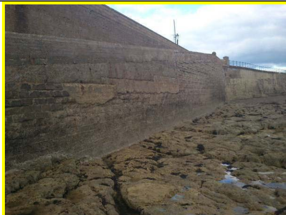
Surface abrasion damage to wall adjacent to ramp showing multiple previous repairs. (Asset ref. No. 1221C901C0303C04)
