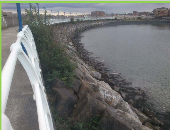
South Pier rock armour on inner face, with vegetation that should be removed. (Asset ref. No. 1221C901C0401C32)
