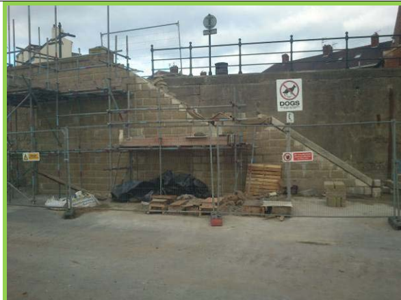
Cracks through deck and crest wall. (Asset ref. No. 1221C901C0401C34)
