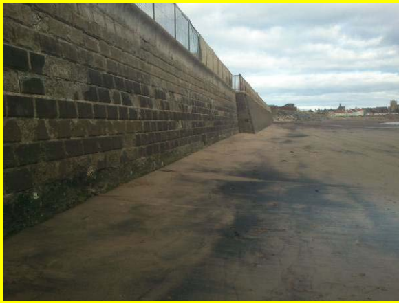
Older concrete block wall in foreground; newer slightly sloping smaller block wall in distance. (Asset ref. No. 1221C901C0401C19)
