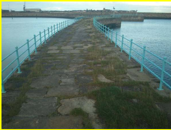
Vegetation growing in between masonry slabs and patch repairs in deck of Middle Pier (Asset ref. No. 1221C901C0401C28)
