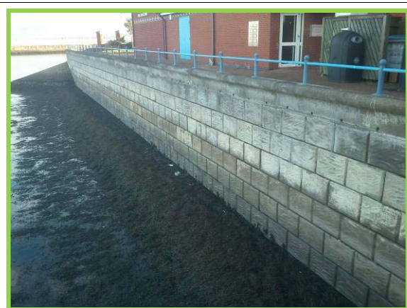
Wall to south side of lock entrance, toe apron covered in seaweed. (Asset ref. No. 1221C901C0401C25)
