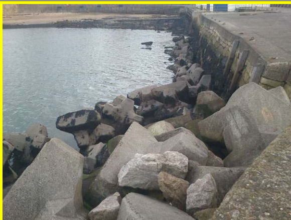
Landward side of Old Pier showing settlement in the (original?) masonry blockwork. (Asset ref. No. 1221C901C0401C06)
