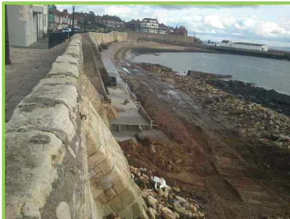
Toe protection apron works underway at Town Wall, (Asset ref. No. 1221C901C0401C35)
