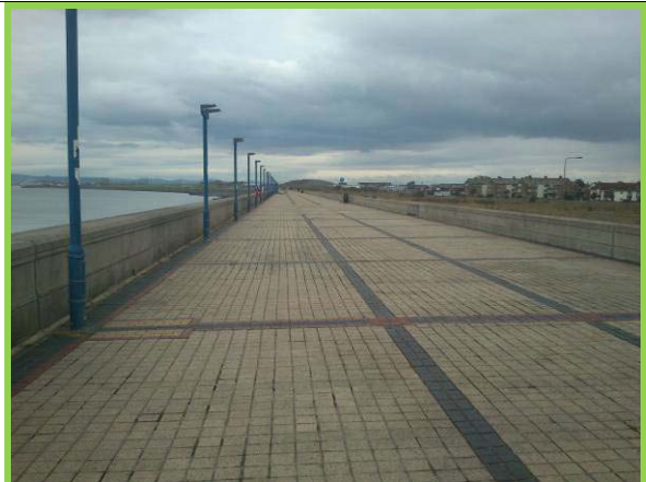
Promenade with crest wall to left and low flood wall to rear (Asset ref. No. 1221C901C0401C33)
