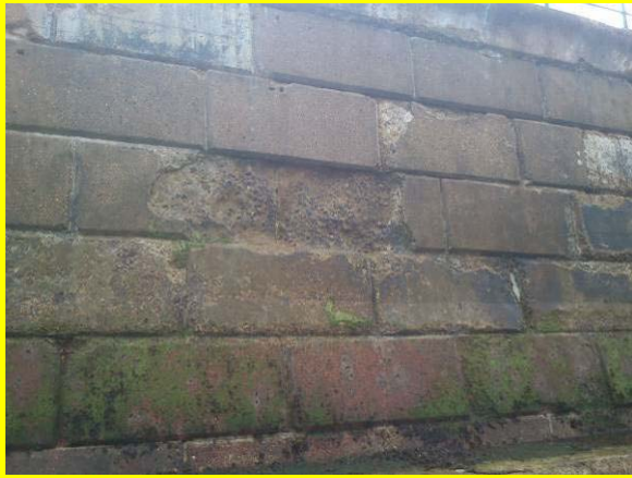
Loss of facing of concrete blocks. (Asset ref. No. 1221C901C0303C02)
