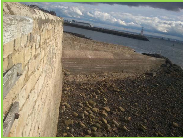
Large groyne structure near mid point of Town Wall marks large change in beach levels. (Asset ref. No. 1221C901C0401C35)
