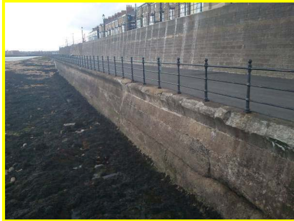
Spalling and damage to coping of front wall (Asset ref. No. 1221C901C0401C05)
