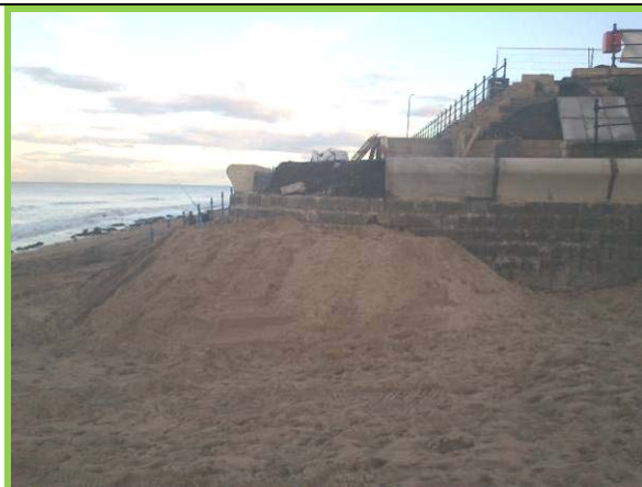
Works underway to replace sections of seawall at return end (Asset ref. No. 1221C901C0303C01)
