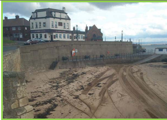
Masonry wall at south east end of Town Wall. (Asset ref. No. 1221C901C0401C35)
