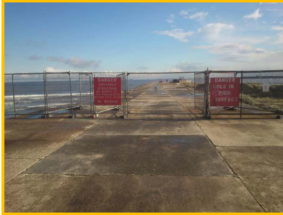
Fencing and warning signs on North Gare breakwater. (Asset ref. No. 1221C901C0502C01)
