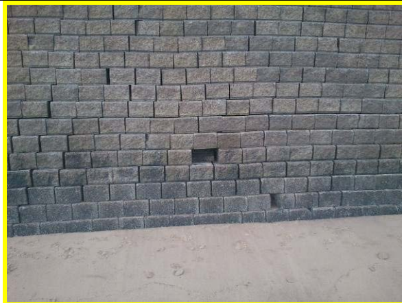
Missing blocks and opening joints (Asset ref. No. 1221C901C0401C19)
