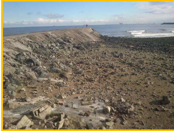
Rubble / slag beach to the south side of North Gare Breakwater. (Asset ref. No. 1221C901C0502C01)
