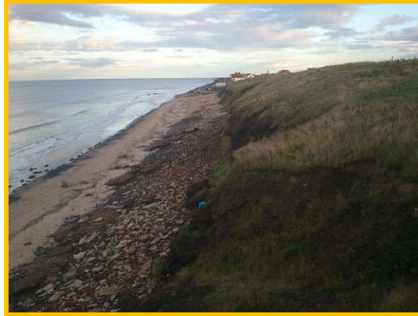
Eroding slag embankment to north west of Marine Drive. (Asset ref. No. 1221C901C0302C03)
