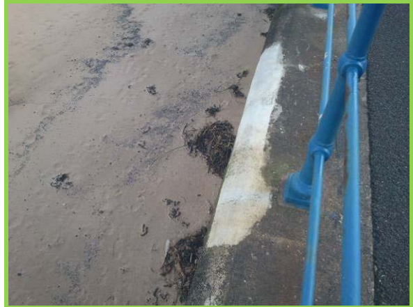
Patch repairs to coping on Marine Drive holding well. (Asset ref. No. 1221C901C0303C01)
