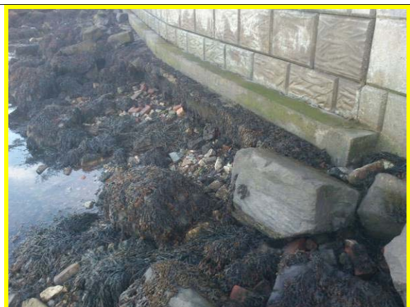
Exposure of wall toe at gaps in toe armour (Asset ref. No. 1221C901C0401C27)
