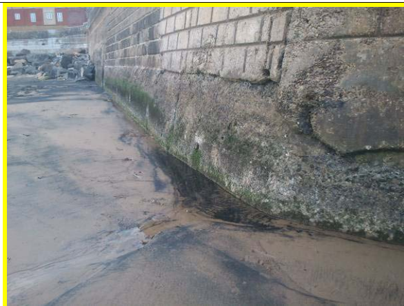
Toe scour and abrasion damage at corner of wall (Asset ref. No. 1221C901C0401C19/20)
